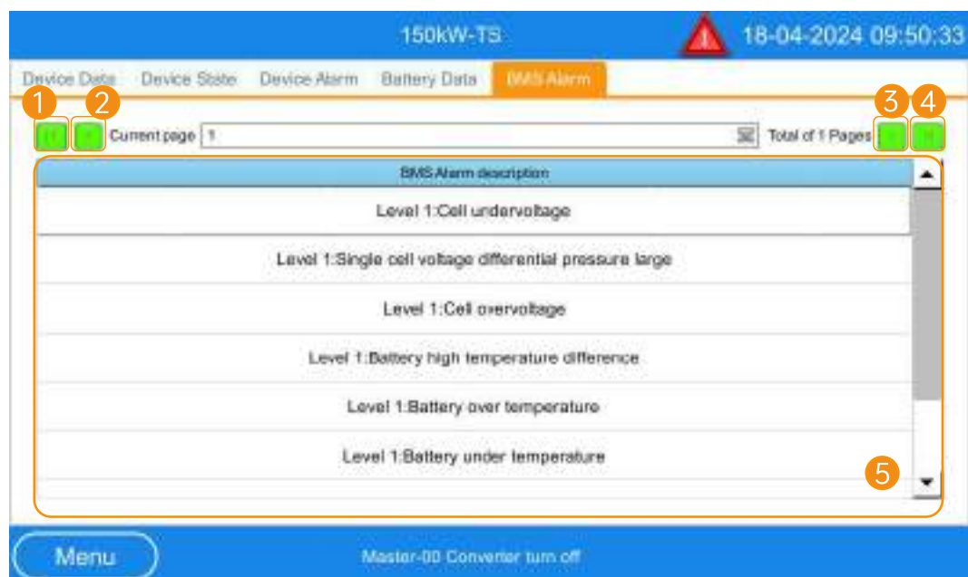
BMS alarm interface introduction
